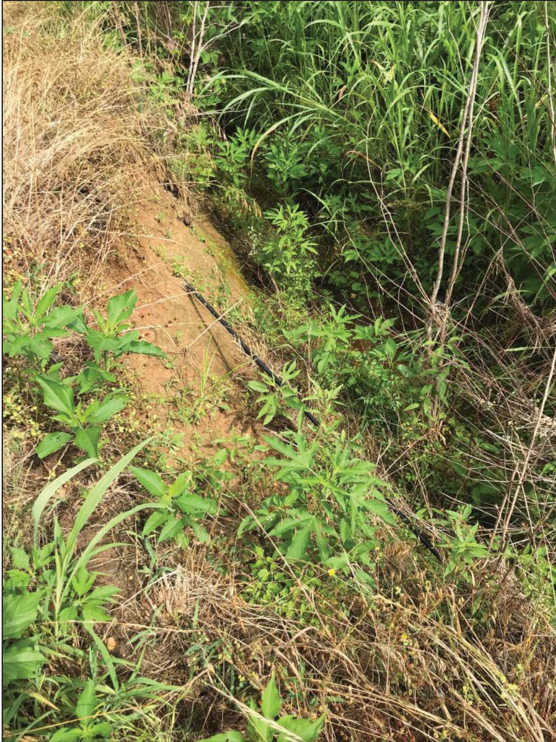
Figure 12. View of Eastern Macon Road APE within the existing ROW, showing erosion and exposed utility cable, View North.
