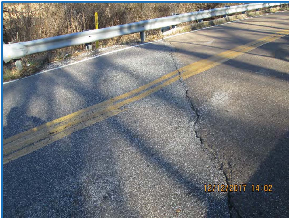
Pavement failure at west end of bridge
